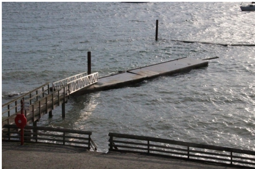
Swimming float and ramp at Armours Beach left unsecured and vulnerable to damage.
